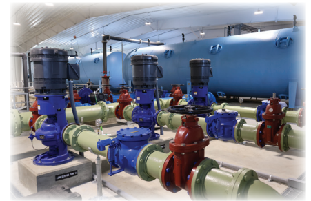
Inside the new Water Treatment Facility.
